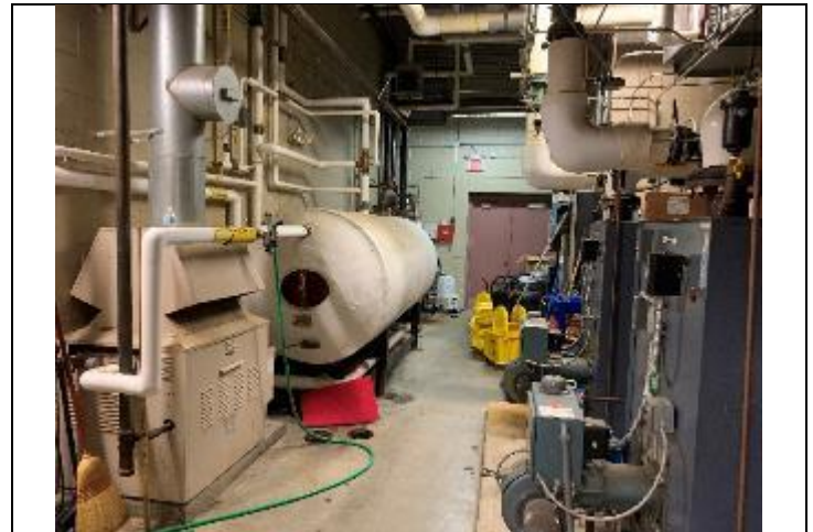
10. Boiler room water tank insulation. No asbestos detected.
