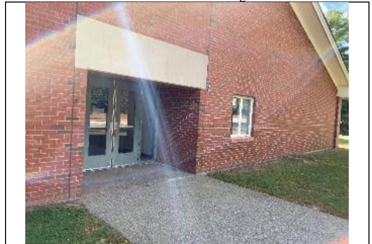
4. Small Entry overhang with gypsum and joint compound as well as door caulk.
